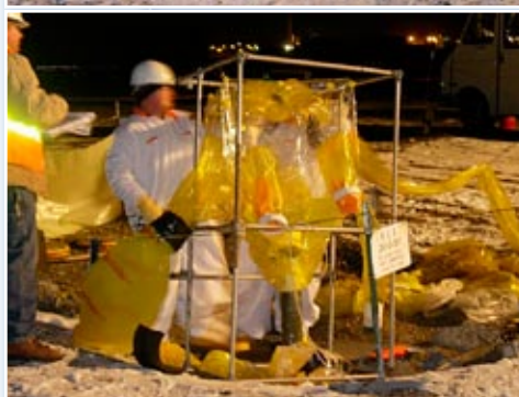
Carefully using measures to control contamination, workers insert a camera through a riser (all photos) in Tank U-361.
